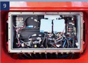
Electrical control system
