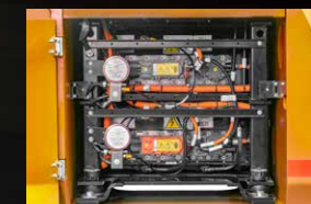
Battery and motor radiator
